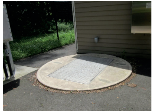
Permit required confined space danger sign not posted at a water pollution control facility wet well entrance.
