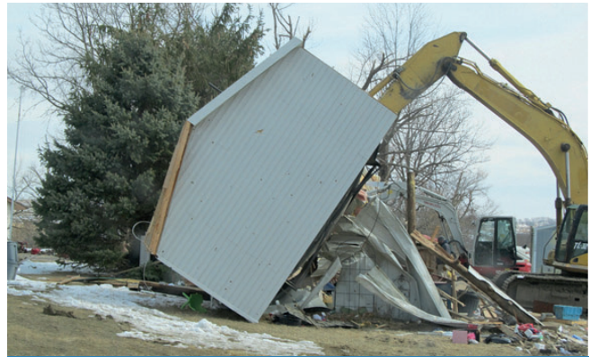
Tornado damage cleanup Winterset, Iowa
