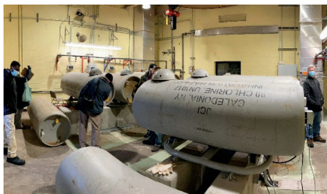
The inside of a large municipal waste water treatment plant with potentially dangerous issues within its chlorine system
