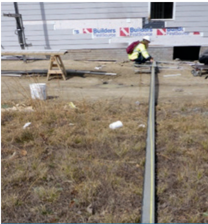
Depiction of the VOSH Compliance Safety and Health Officer taking measurements of the pole that contacted the overhead powerline.
