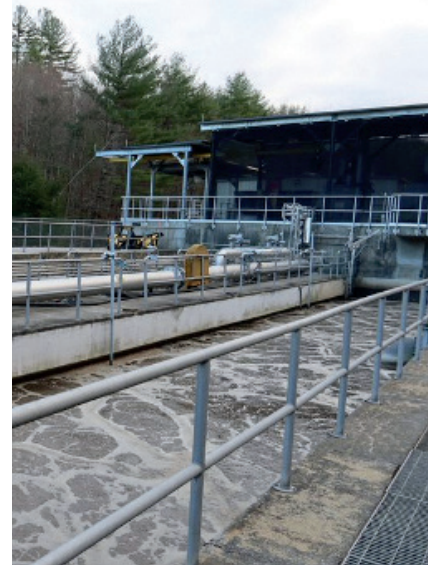
Rails at the water pollution control facility are not compliant with fall protection requirements.
