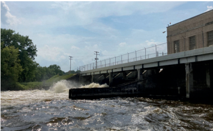
The powerhouse section of the Calkins Bridge Dam showing the intensity of the spillway flow and choppy, murky, and turbulent current awaiting the divers on July 7, 2021.
