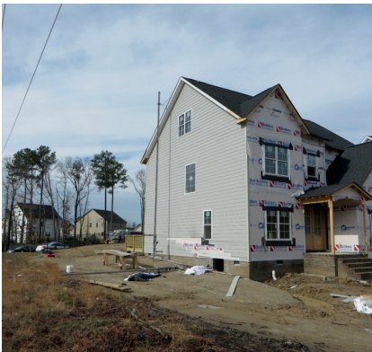
Location of the scaffold's pole that contacted the overhead powerline laying on the ground.
