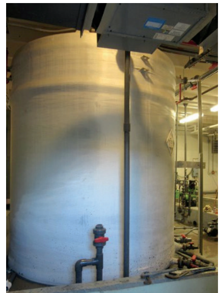
One of two 3,000 gal. sodium hypochlorite tanks involved in uncontrolled release at water treatment plant.
